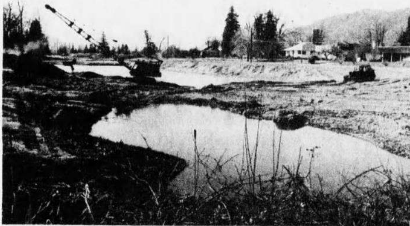
Heavy equipment section of Base Transport shown near completion of the Bell Slough project on Fairfield Island. In this project approximately 20,000 cubic yards of material were moved to make way for a senior citizens park.
