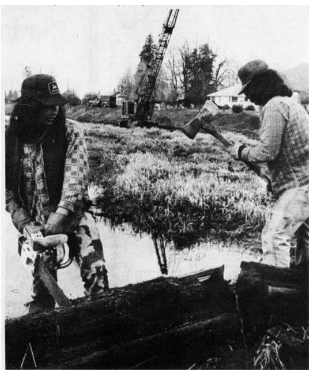
FROM SLOUGH TO FISHING SPOT — Chilliwack Rotary Club's Bell Slough project will transform this section of the waterway into a community park and fishing spot. Workers for the project have been supplied through a federal government Local Initiatives Program grant. The drag line was provided by CFB Chilliwack.
